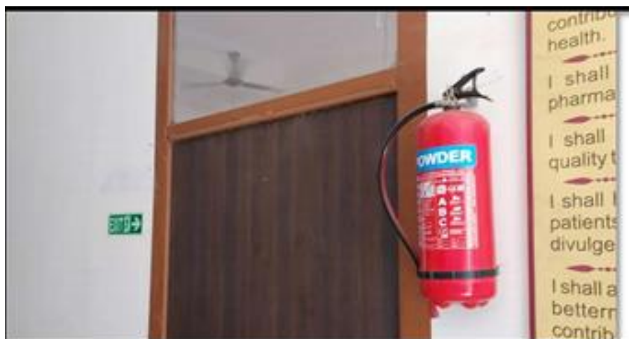
Fire Fighting System is installed
