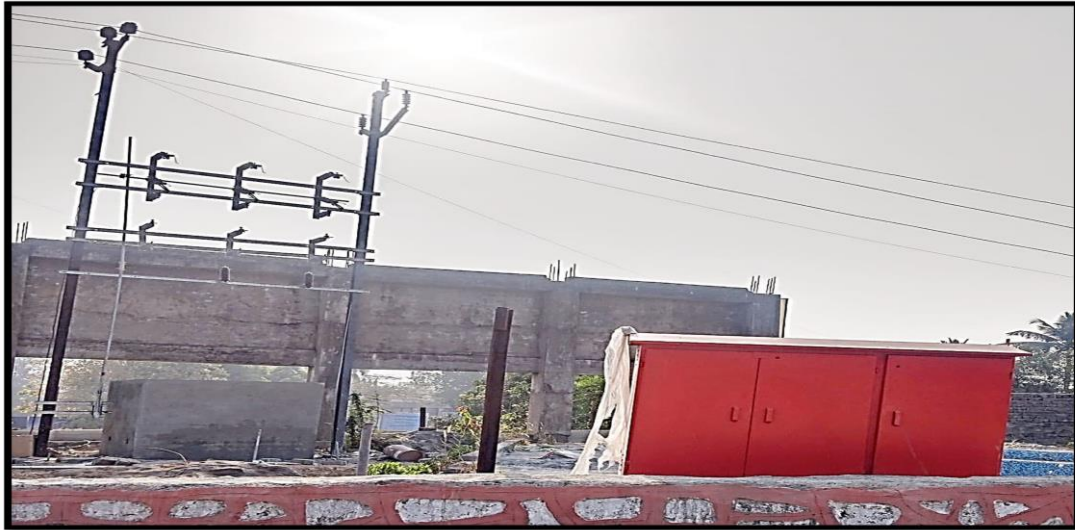
FIGURE. TRANSFORMER INSTALLED IN 2024
